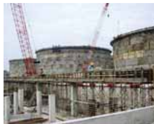
Civil and Related Works for Tank Foundation and Other Structures at the Land next to Meranti Crescent - MK No 34 at Jurong Island
