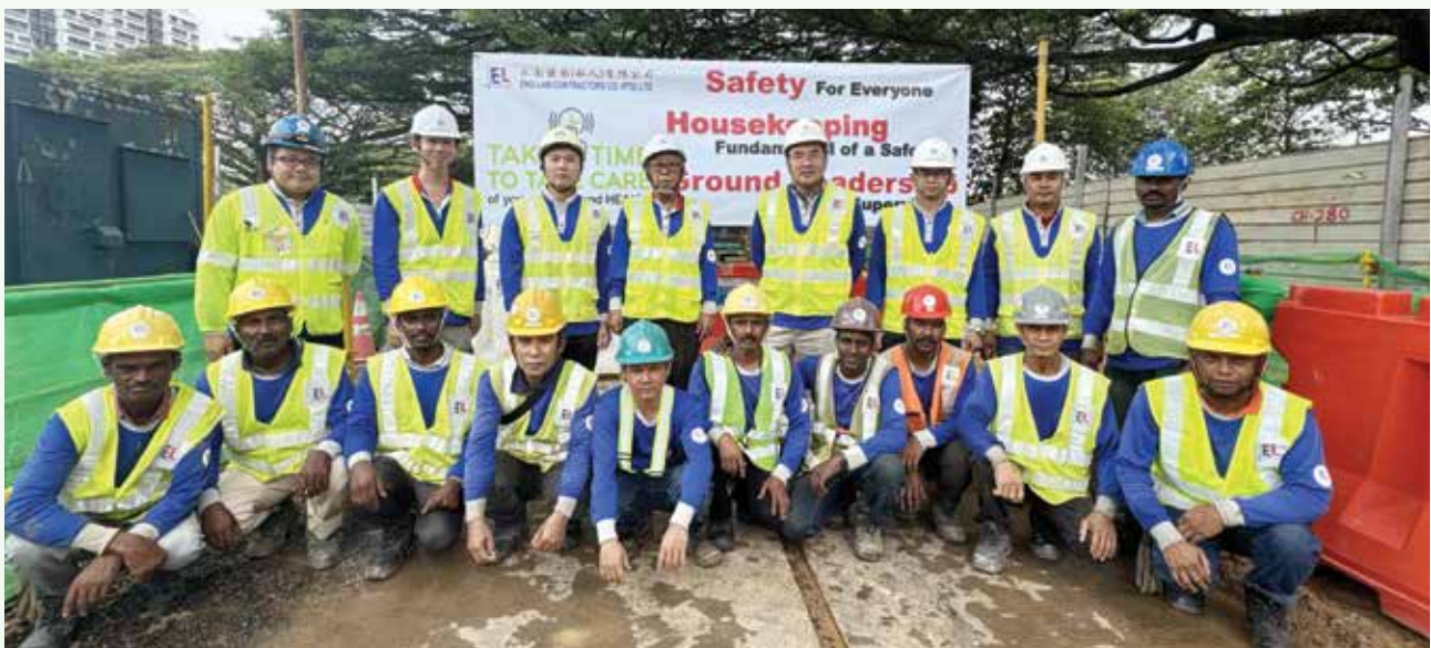
Ensuring good safety and housekeeping standard at one of OKP's project sites.
