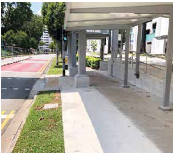
OKP is involved in the ongoing construction of covered linkway at Woodlands.
