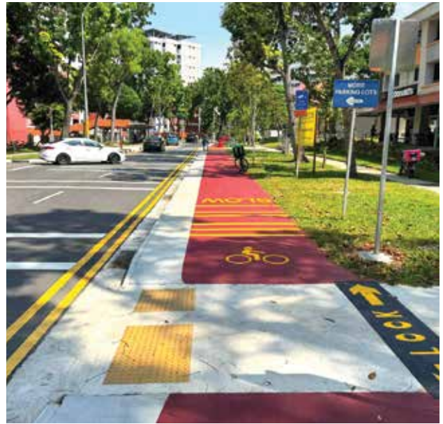
OKP is involved in the construction of the Cycling Path Network at Kaki Bukit- Bedok Reservoir.
