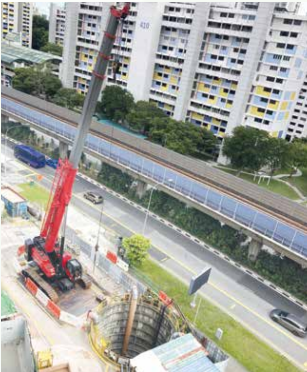
Deep Tunnel Sewerage System at Commonwealth Avenue 2 is an OKP's ongoing project.
