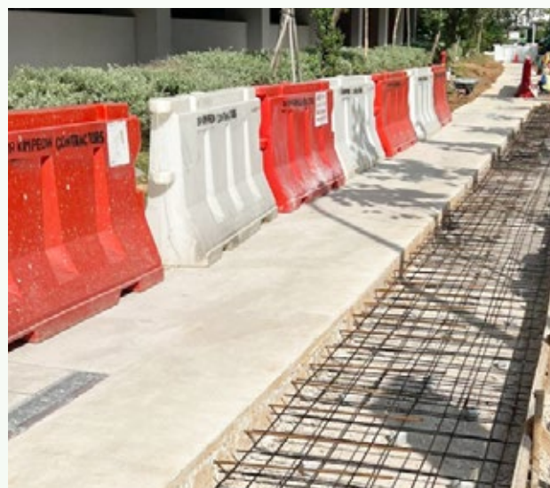
OKP is exploring the use of Glass Fibre Reinforced Polymer, which is on trial at Potong Pasir.
