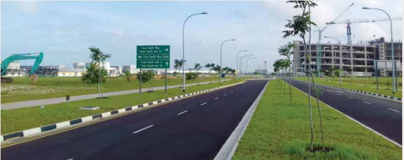
OKP is involved in the construction of roads, drains, sewers and soil improvement works at Tuas South Avenue 7/14.
