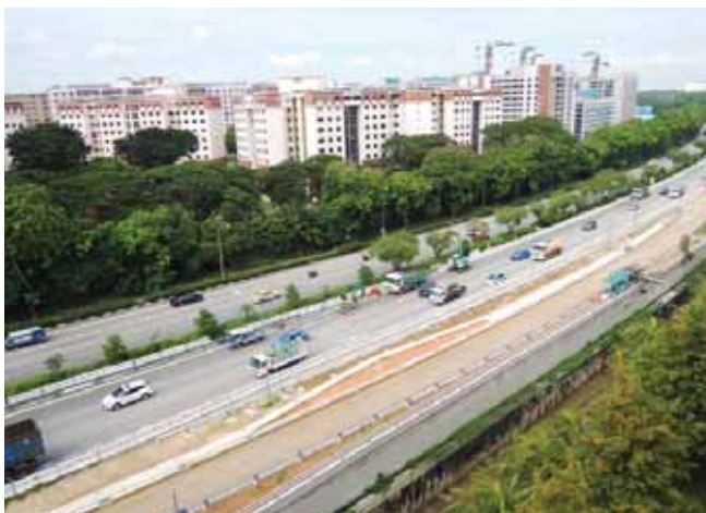
OKP is involved in the construction of the viaduct from TPE to PIE (Westbound) and Upper Changi Road East.
