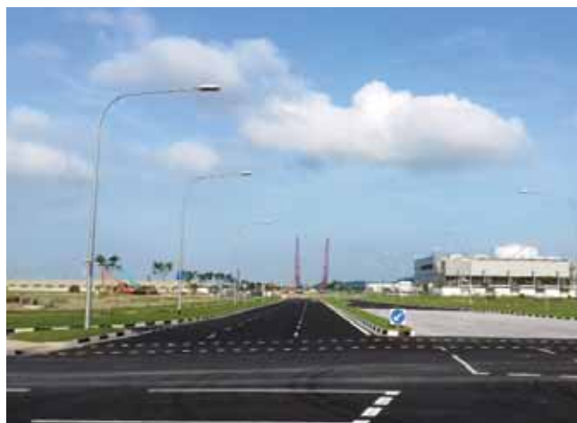
OKP is involved in the construction of roads, drains, sewers and soil improvement works at Tuas South Avenue 7/14.
