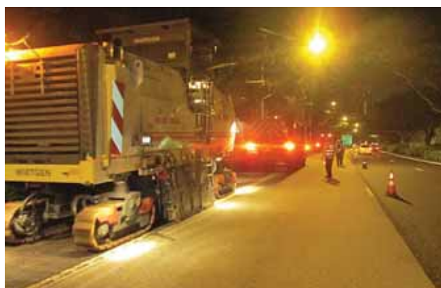
Road resurfacing works along ECP, SLE, BKE, CTE and KPE being carried out at night.
