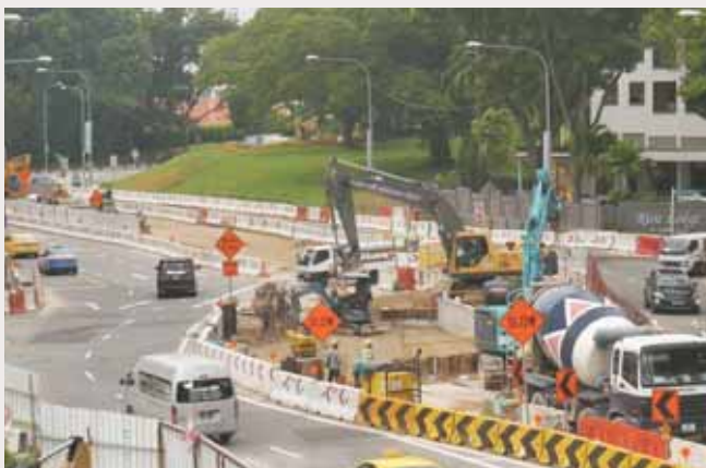
The construction of Stamford diversion canal – Tanglin and Kim Seng by OKP.
