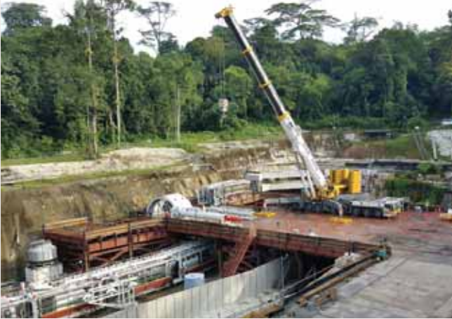
Improvement to Bukit Timah first diversion canal from Holland Road to Clementi Road by Chye Joo - Or Kim Peow JV.
