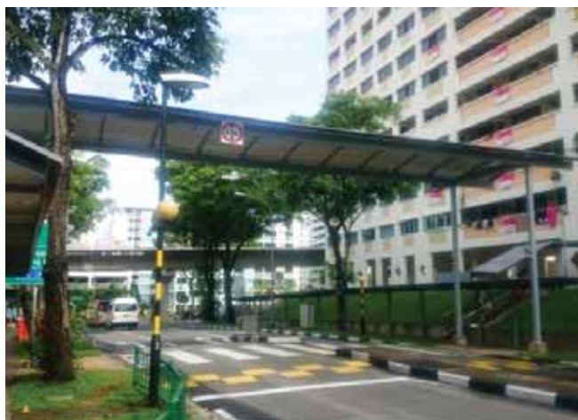
OKP build a high-covered linkway at Bangkit LRT in the Walk2Ride programme (ER442).
