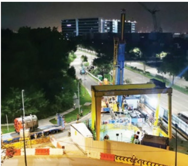
OKP is involved in the construction of link sewers from the Deep Tunnel Sewerage System phase 2 project – schedule III contract 1 (Jalan Buroh/Tanjong Kling Road).
