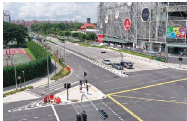
Commuter and road infrastructure works in Pasir Ris and Loyang is an OKP's ongoing construction project.
