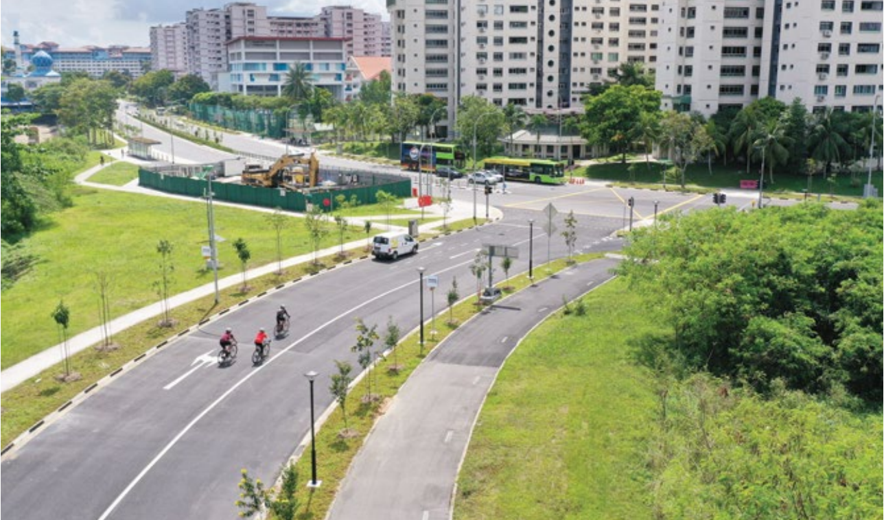
One of OKP's ongoing construction projects involves commuter and road infrastructure works in Pasir Ris and Loyang.
