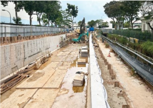
Improvement to Sungei Selarang and its subsidiary drain A is an OKP's ongoing construction project.
