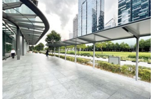
OKP is involved in the Shenton Way Station under the construction of covered linkways to Thomson East Coast Line (TEL) Stage 1, 2 and 3 Stations.
