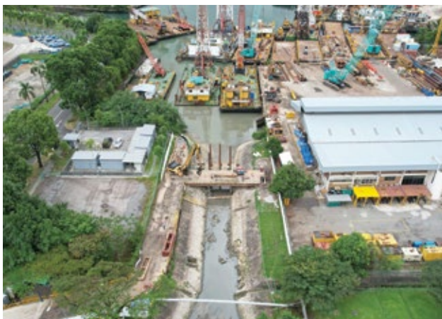
One of OKP's ongoing construction projects is the improvement to Benoi Road outlet drains.
