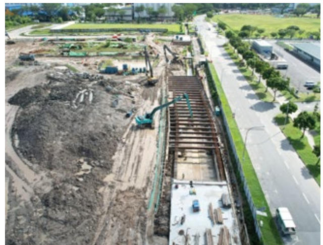
Proposed construction of new infrastructure at Tukang Estate is an ongoing OKP's construction project.
