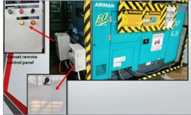
Physical setup of autostart generator.
