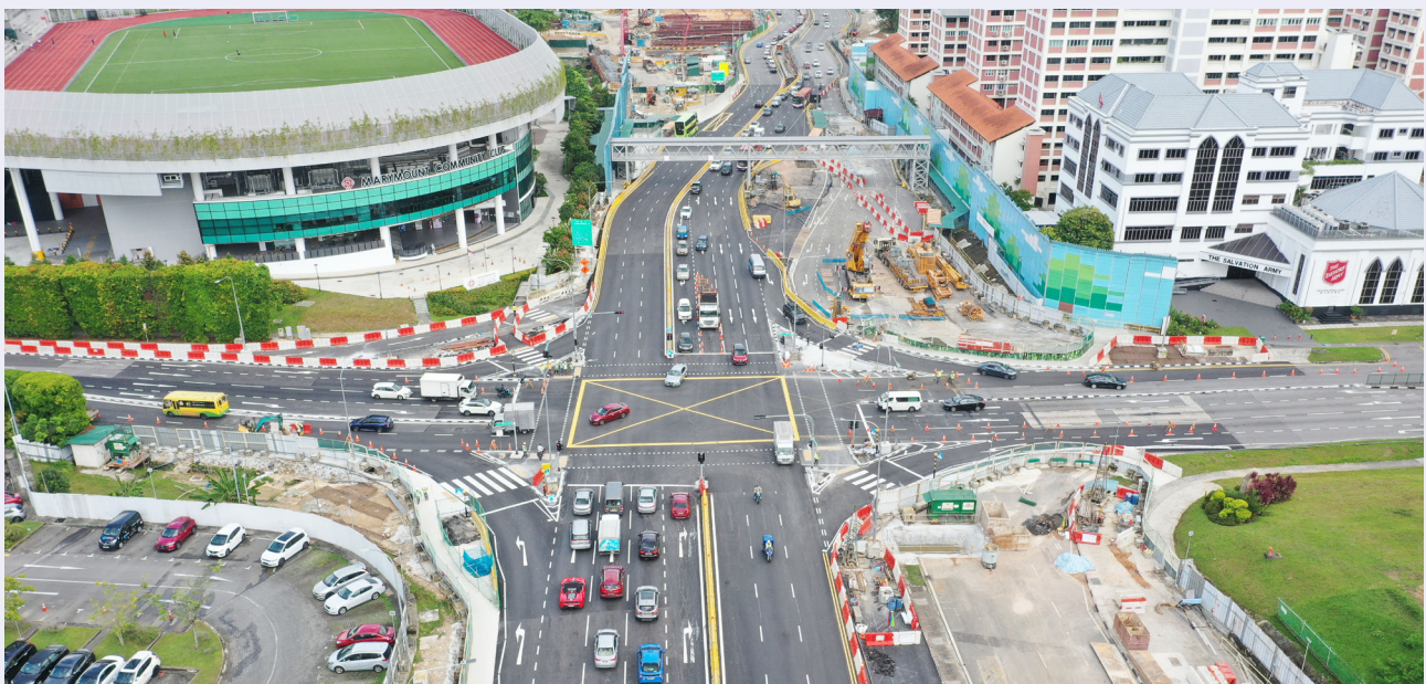
One of OKP's associate companies is involved in the design and construction of the North-South Corridor (Tunnel) between Pemimpin Place and Sin Ming Avenue at Marymount Junction.
