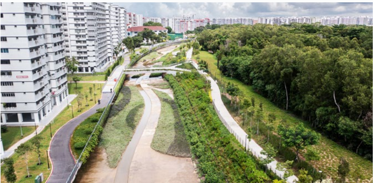
One of OKP's construction projects involves the improvement to Sungei Tampines (Tampines Avenue 7 to Tampines Expressway).
