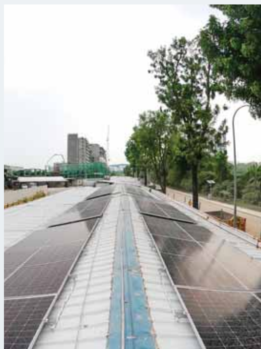
Photovoltaic system at Jalan Papan office.
