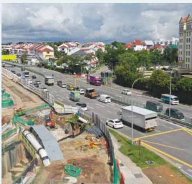
Bored piling works at Loyang Avenue is an OKP's ongoing construction project for commuter and road infrastructure works in Pasir Ris and Loyang.
