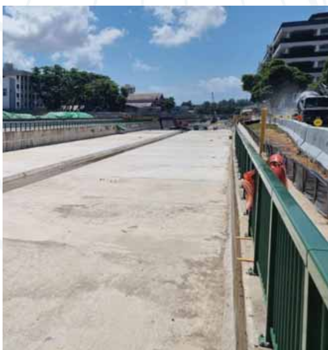
Improvement to Sungei Selarang and Sungei Selarang subsidiary drain A is an ongoing OKP's construction project.
