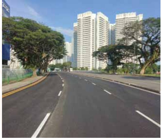
OKP is undertaking road maintenance for South East Sector at Upper Boon Keng Road.
