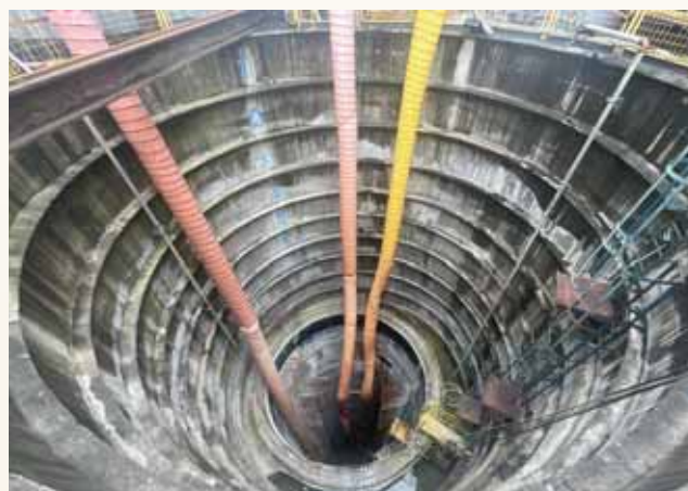
Construction of link sewers for the Deep Tunnel Sewerage System Phase 2 project at Tanjong Kling Road is one of OKP's ongoing construction projects.
