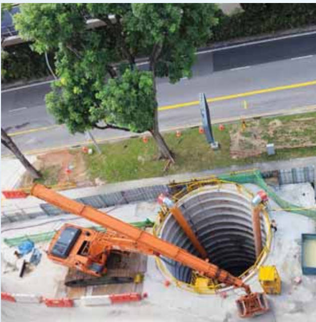
OKP is involved in the construction of link sewers from the Deep Tunnel Sewerage System at Commonwealth Avenue.
