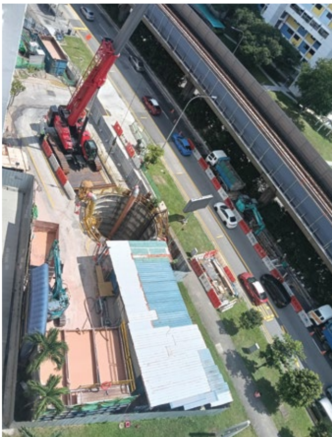
Construction of link sewers for the Deep Tunnel Sewerage System Phase 2 project at Commonwealth Avenue is an OKP's ongoing construction project.
