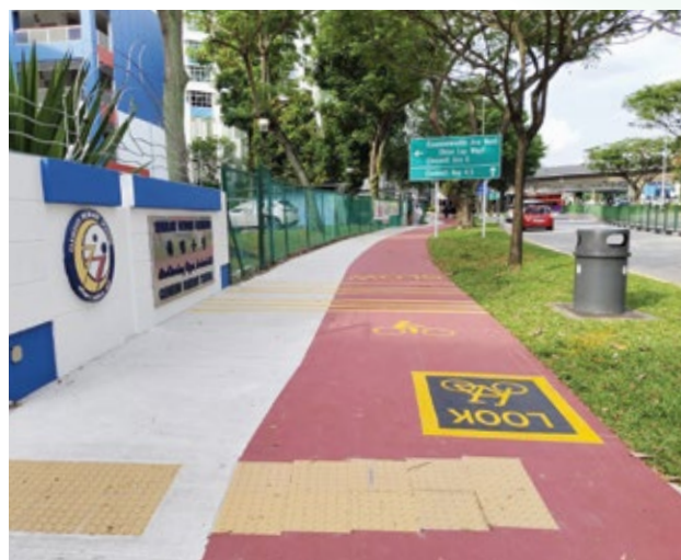
Construction of Cycling Path Network West at Clementi Avenue is an OKP's newly awarded project.
