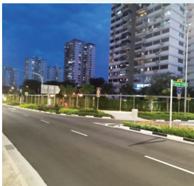
Commuter infrastructure enhancement at linkway at Siglap MRT is an ongoing OKP's construction project.
