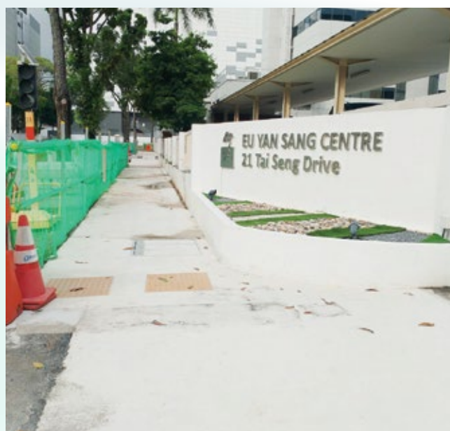
OKP is involved in the improvement to roadside drains at Eng Kong Place.
