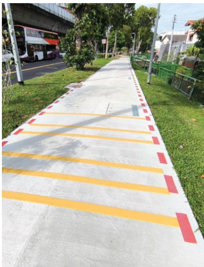
Resurfacing work at New Upper Changi Road is one of OKP's footpath renewal maintenance projects.
