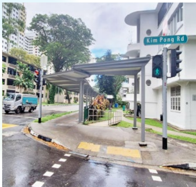
Construction of covered linkways at Havelock Road to Thomson East Coast Line (TEL) Stage 1, 2 and 3 Stations is an OKP's ongoing construction project.
