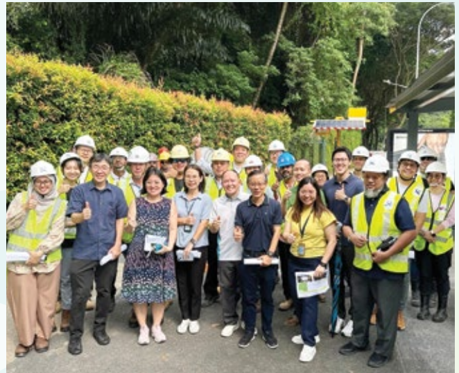
LTA Active Mobility Group Director Mr Chan Boon Fui (second from left) visited the site for the construction of Cycling Path Network (Central) on 24 October 2024.
