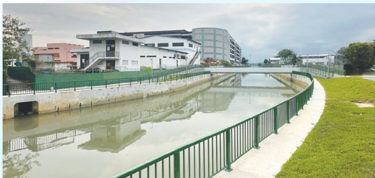
OKP is undertaking the improvement to Sungei Selarang and Sungei Selarang subsidiary drain A project.
