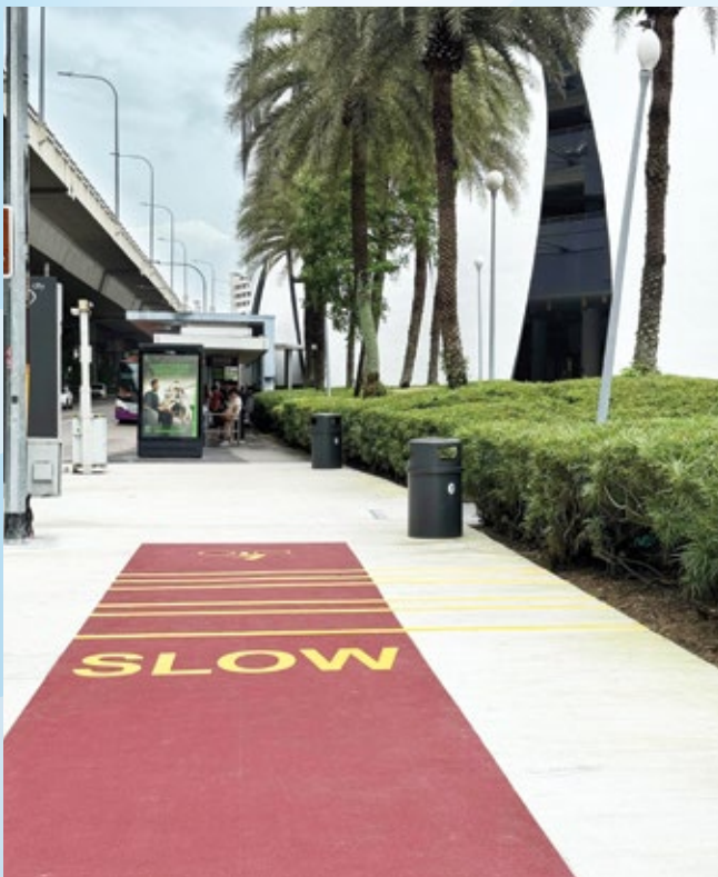
Ongoing construction of Cycling Path Network (Central) at Vivocity, which is an OKP's newly awarded project.
