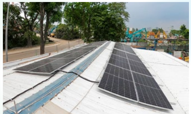
Photovoltaic system at Jalan Papan project site office.
