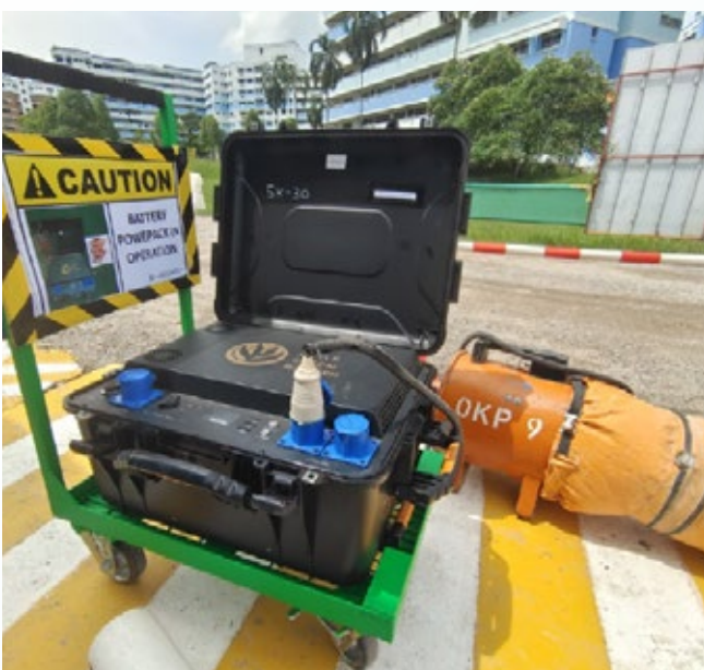
This eco-friendly power pack provides clean and efficient energy at OKP's project sites.
