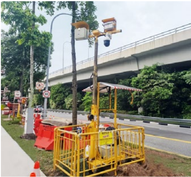
OKP relies on solar panels to power the CCTV cameras at all OKP's project sites.
