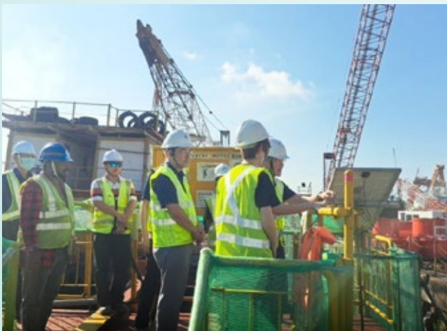
PUB Senior Deputy Director Lim Joo Hsien Albert visited an OKP's construction site.
