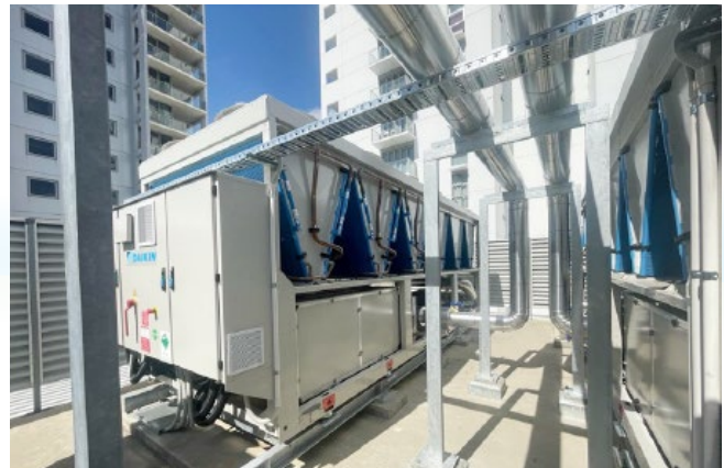
Replacing existing chillers with energy-saving models that can significantly reduce energy consumption and operational costs at 6-8 Bennett Street, East Perth in Australia.
