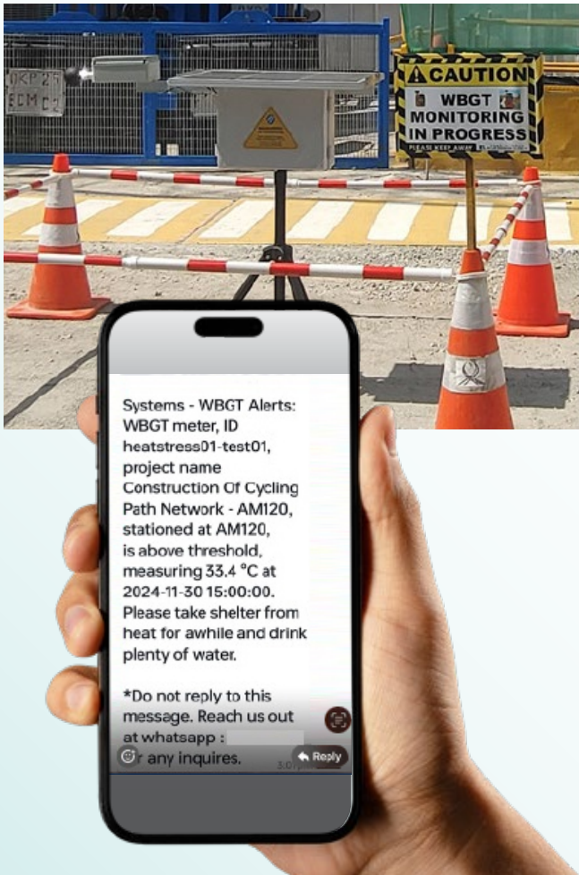
Real-time WBGT monitoring and auto alert system.
